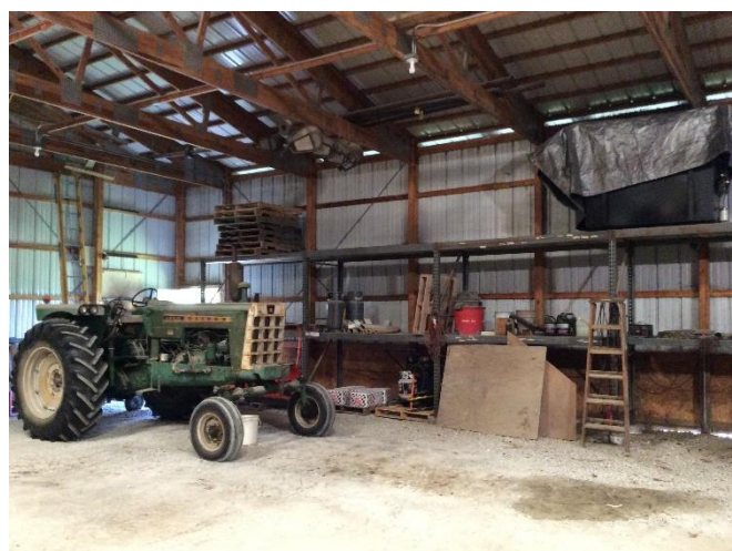
16. De minimis surface staining from tractor storage observed in the Pole Barn.
